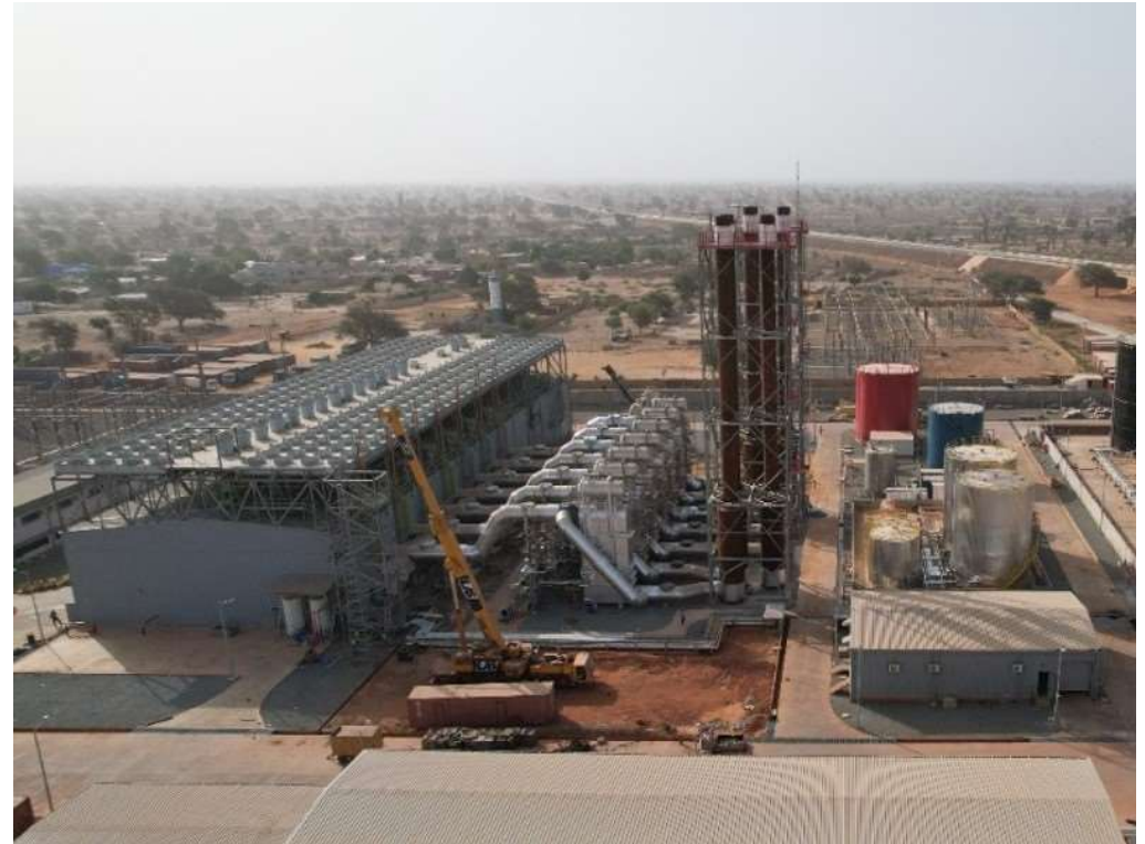
130 MW Malicounda Power Plant, Senegal
